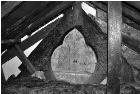
Figure 5. 45 Mill St, Leominster. The apex of the smoke blackened cruck truss over the middle of the former hall showing the quatrefoil decoration and the shallow angle of the later, raised roof.
