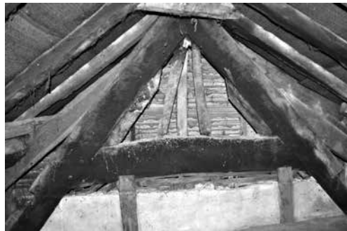
Figure 6. 45 Mill St, Leominster. The truss at the west end of the former hall which uses the wallplate of the lost crossing for a tie-beam. Note the upper edge of the principal rafters where the thatch on the original roof has kept the timber clear of smoke blackening.
