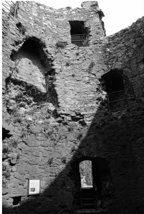
Figure 7. Dundrum Keep: interior showing modern ground-floor entrance, first-floor hall with fireplace and chimney, internal openings to spiral staircase at ground, first and second floor, and wall walk.
