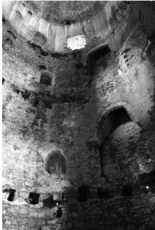
Figure 10. Pembroke keep showing joist holes on ground, first and second floors, two fireplaces and interior of domical roof.
