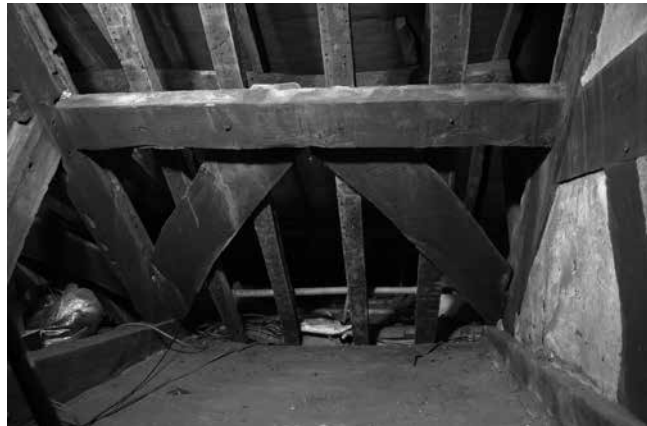
Figure 3. The roof of the cross passage bay of the hall range within The Hop Pole. This view, looking east, shows the wind braces and the threaded purlin with the primary rafters still in situ, all beneath the protection of an oversailing, later roof
