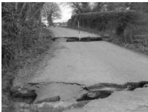
Figure 2. Two of the cracks in the Ullingswick to Pencombe Road
