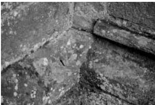
Figure 2. Return in the plinth mouldings between the church porch and the stub of a former north aisle buttress. The porch is on the right
