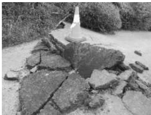
Figure 3. Distortion of tarmac surface caused by the landslide
