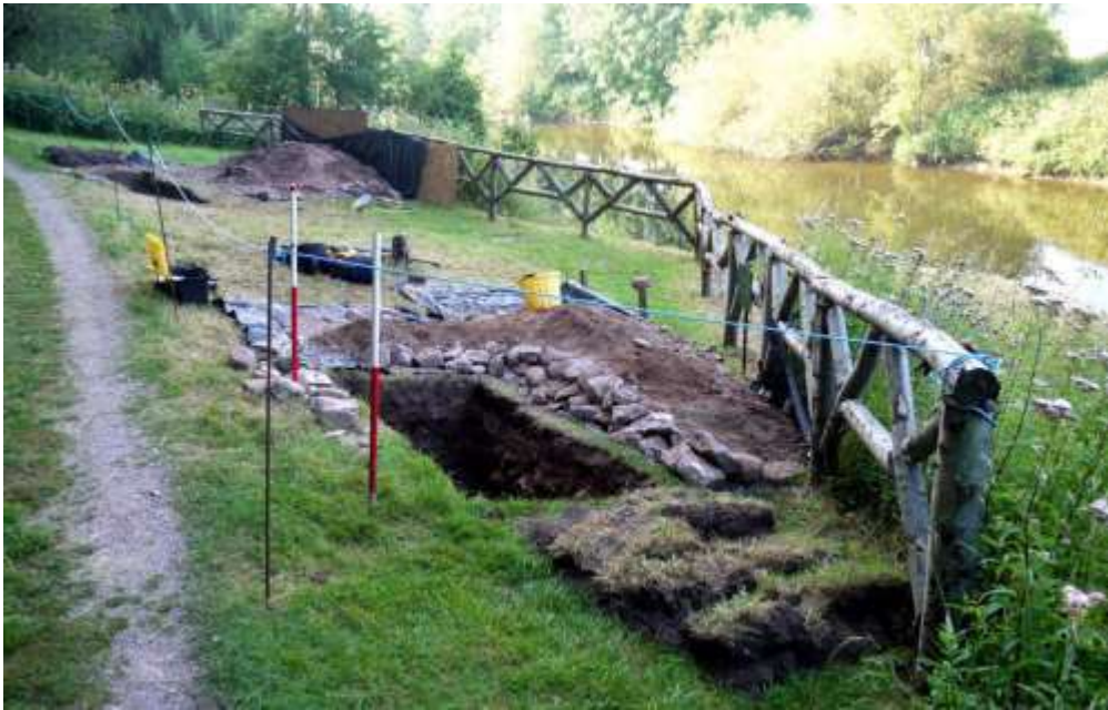
Plate 5.1. New Weir: view south-east across the terrace. Trench 2 in foreground and trench 1 in the background.
