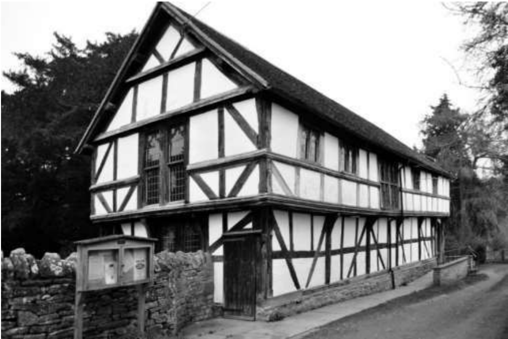
Figure 4. Parish Hall, Cradley. The former church ale house and later a school with its jettied upper storey still in place although the actual floor inside has been removed
