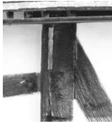
Figure 3. Plugged mortices formerly housing brackets to support the jetties can be seen at the top of the posts along both sides of the building
