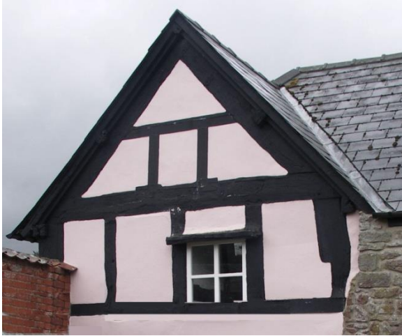
Figure 15. Oriel window before repair
