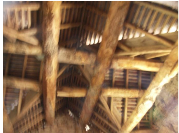
Figure 13. The roof timbers in 2013, taken with difficulty as there was no access to the dovecote.
