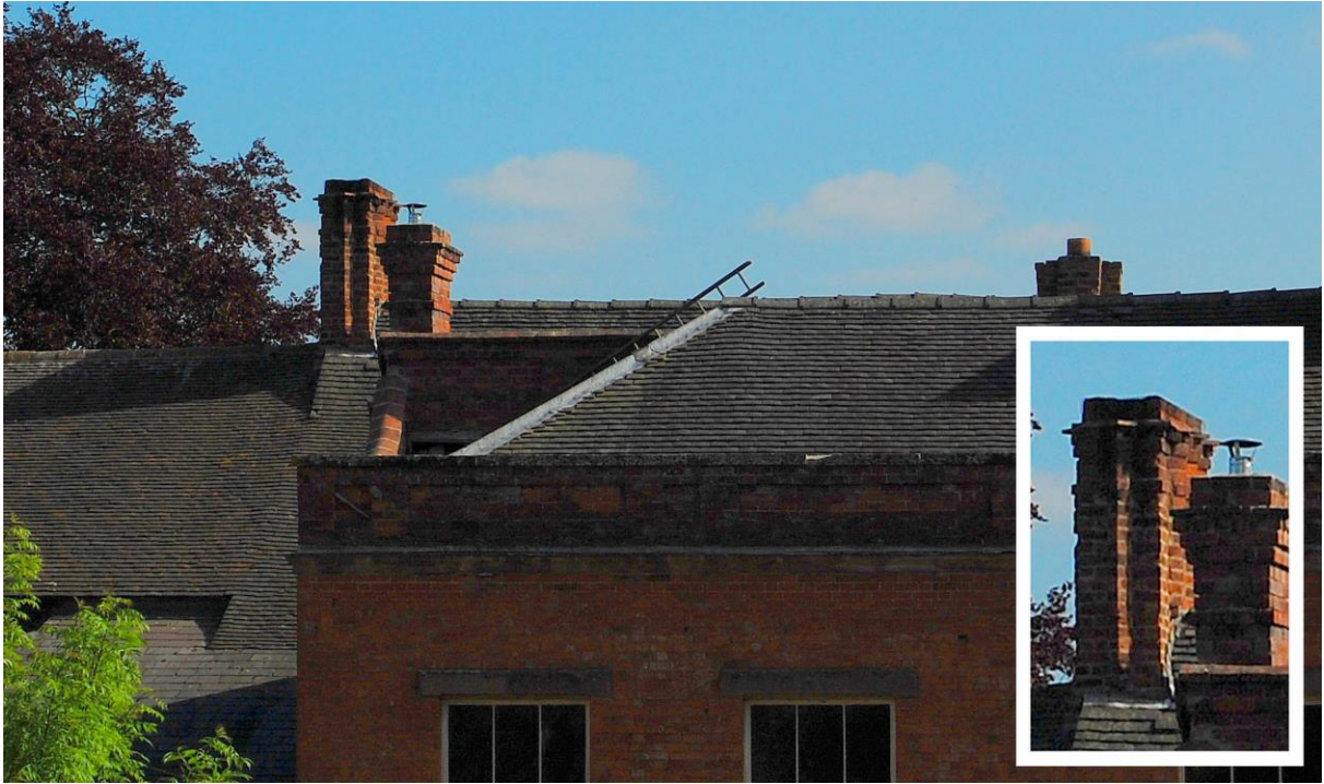
Figure 13. The windows facing the camera lie on the north side of Buckland House. The early chimney on the east side is partially obscured by one of the later chimneys probably built by Mr Cherry.
