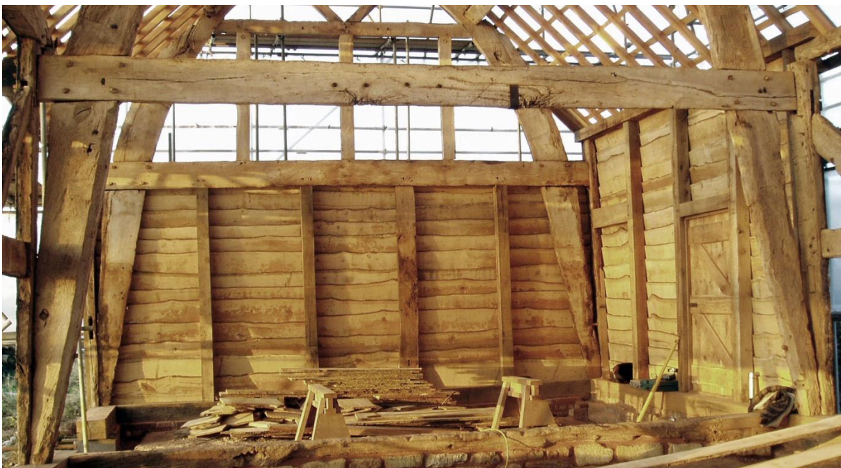
Figure 5. The two most north-westerly cruck pairs seen clearly with the roof off
