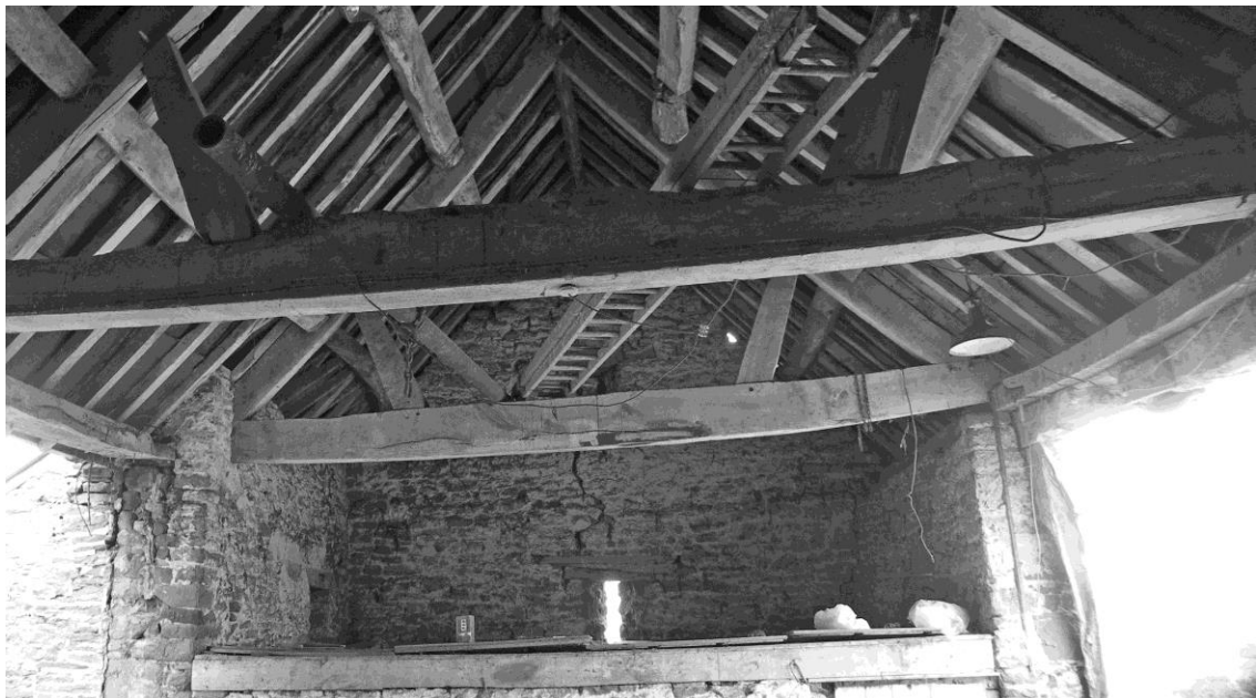
Figure 7. The beams in the threshing barn either side of the threshing floor
