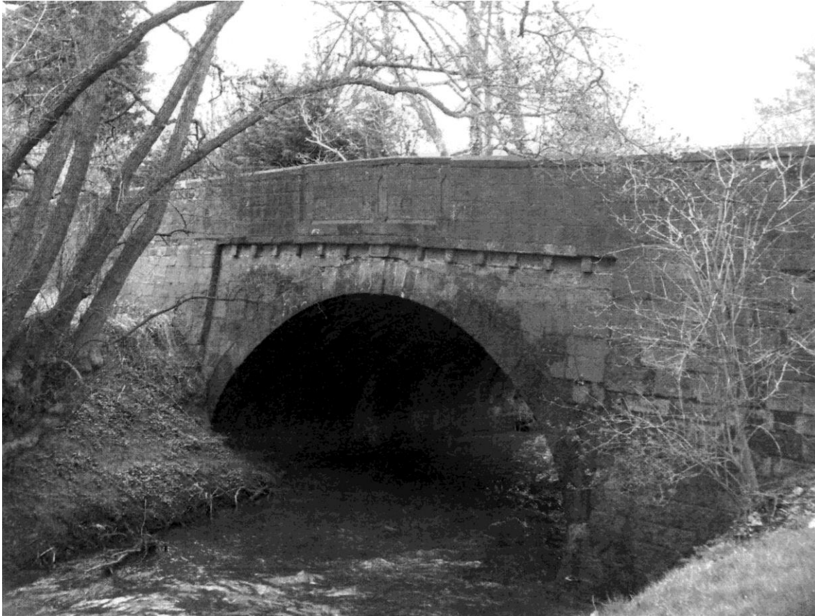
Figure 1. Old Forge Bridge from the downstream side, about 200 metres before the Garron meets the Wye. The other side is decorated identically
