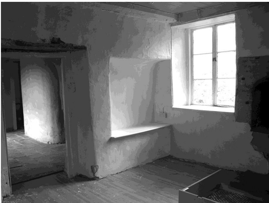
Figure 7. Blocked window between buildings
