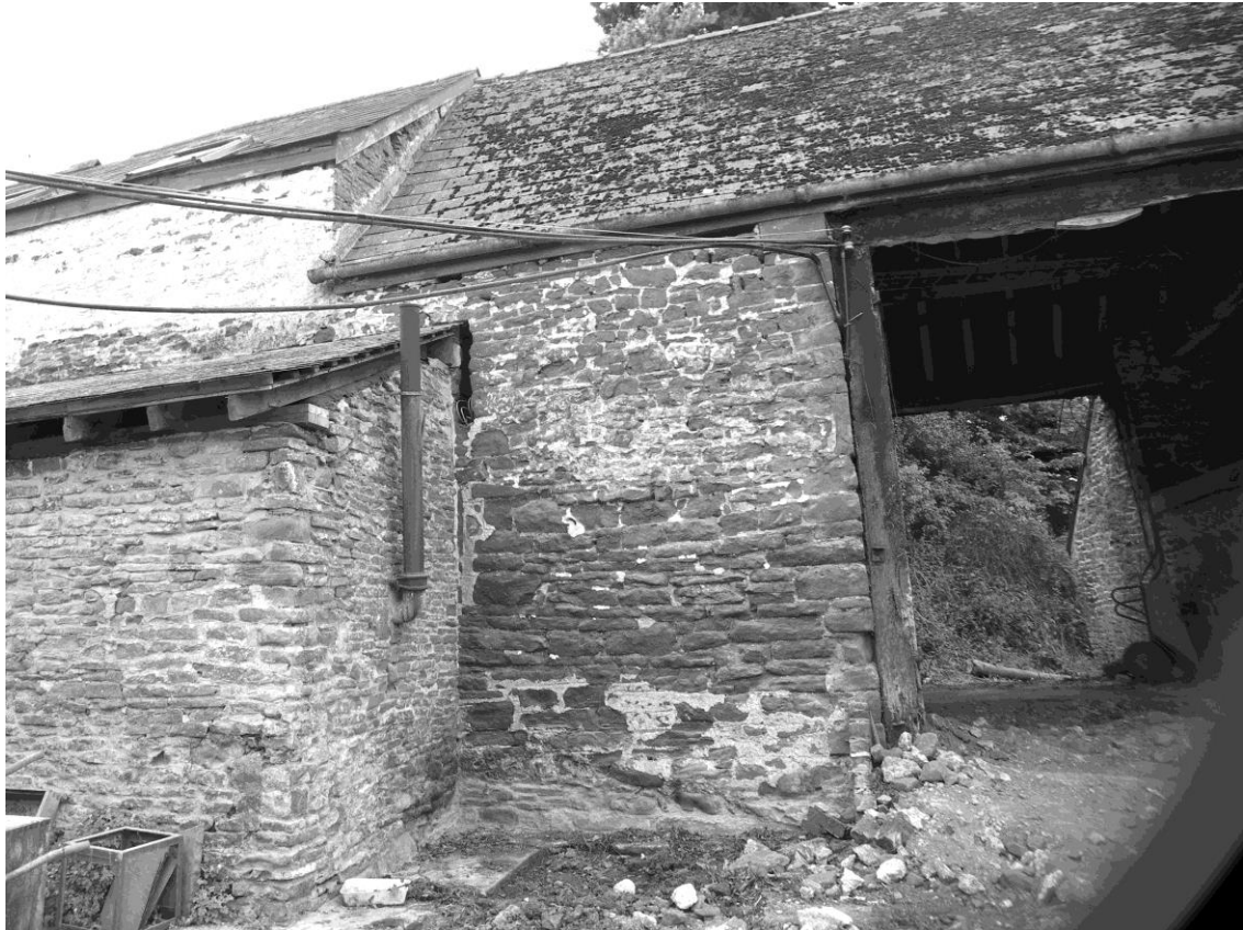
Figure 6. North-eastern side of the threshing barn, at its junction with the newer part next to the house. This gives a fair indication of the various buildings which have been added to the original barn
