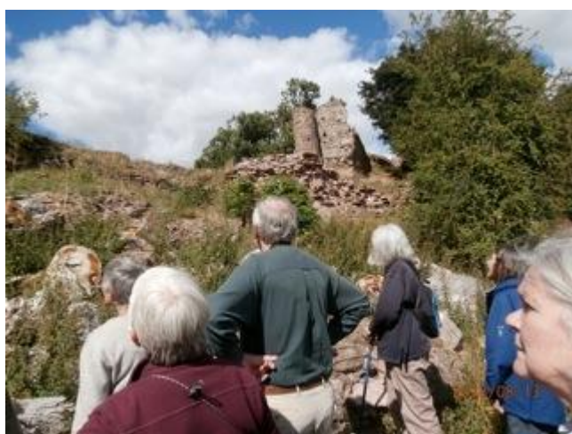
Plate 3: South side of Snodhill Gate Tower and Keep from 12 m below. Inner bailey wall forms skyline on the left.
